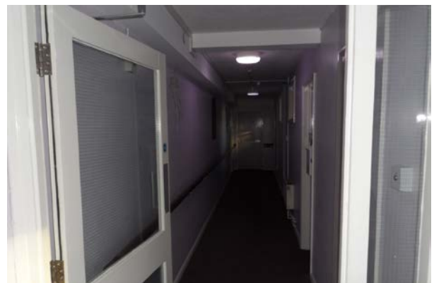
Communal circulation needs redecoration
