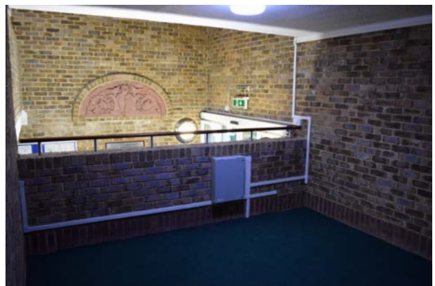
Unused circulation area with poor quality electrical installation.
