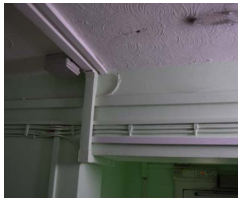
Exposed wiring at Woods House
