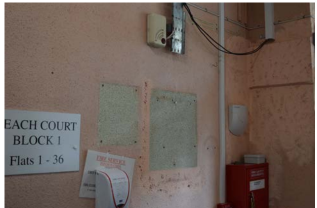
Some communal areas are in poor condition
