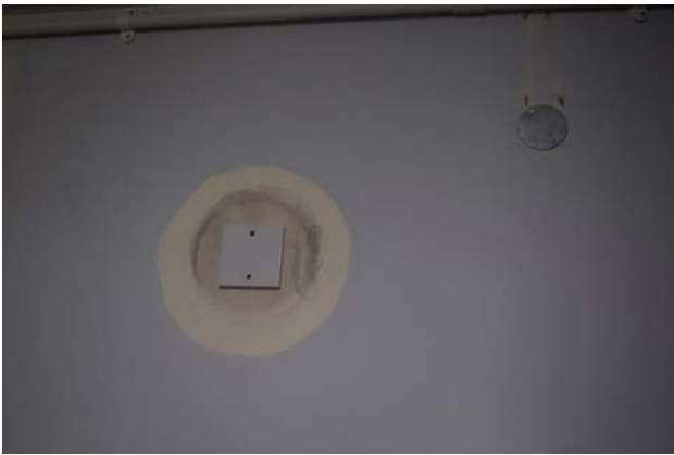
Poor quality repair after the replacement of a light
