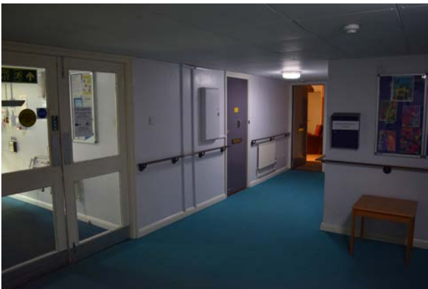
Ground floor flats in close proximity to the main entrance experience noise issues
